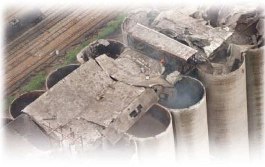
Figure 4.13 This grain elevator blew up when the extremely fine grain dust in the air was ignited accidentally. The fine dust means a large surface area of grain was available for the combustion reaction.
