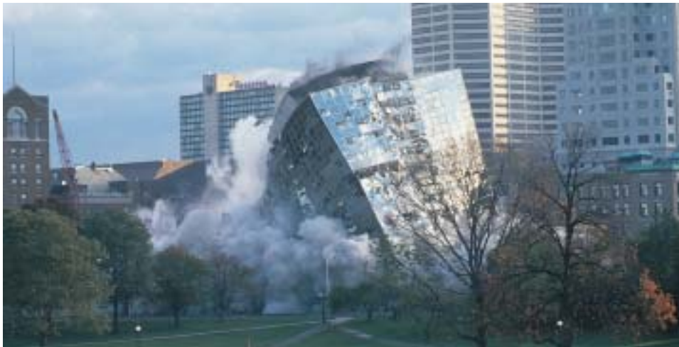
Figure 3.4 Part of the mechanical energy in a building demolition is transformed from the chemical energy of explosives. Much of the energy in the demolition comes from the gravitational potential energy of the building itself. The collapse of the support columns triggers the release of this energy.
