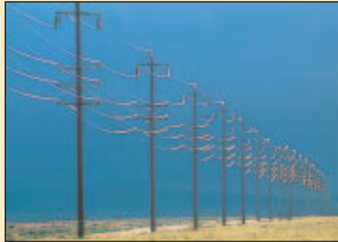
Figure 2.19b) Workers set up these electrical cables during the summer. You'll notice that the cables are not stretched tightly. They sag. What is the advantage of leaving some slack when installing electrical cables like these? What might happen if the cables were installed tightly with no slack?
