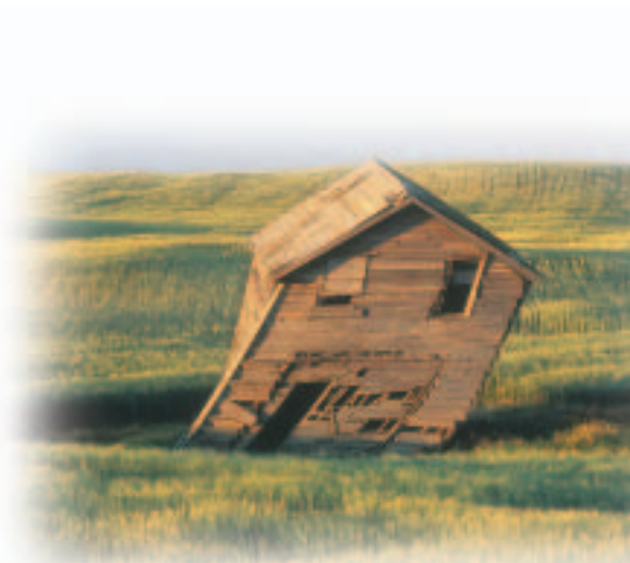
Figure 3.12 No matter how good a structure's design is on the drawing board, the ultimate strength and stability of that structure depend on the right materials and method of joining being used.
